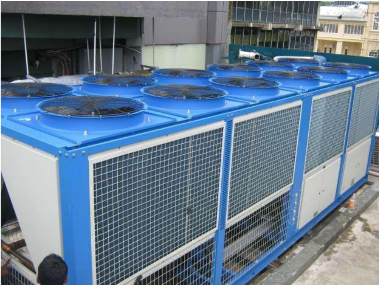
THIS CHILLER IS INSTALL AT ROLALABAU HOUSE
